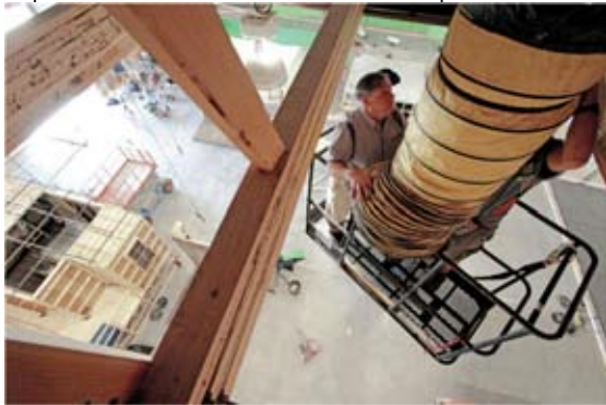
From left, intern Dan Hodges of Albuquerque and Santa Fe Studios employee Max Sinclair remove an air-conditioning duct at the studio on Wednesday. Hodges is a student in the film technician training program at Santa Fe Community College, which requires a hands-on internship in the film industry. Luis Sánchez Saturno/The New Mexican
